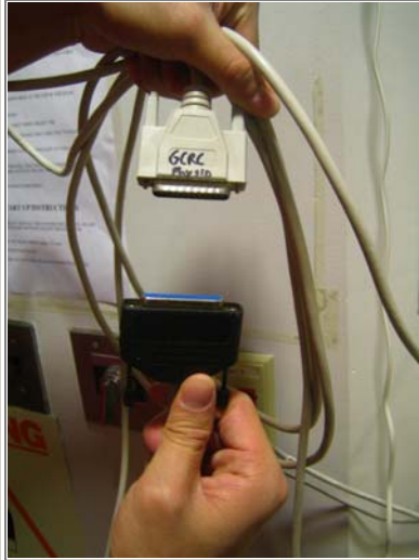
Images 10: DB-25 cables connecting in the control room
