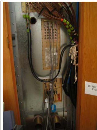
Image 6: The penetration panel in bay 2
